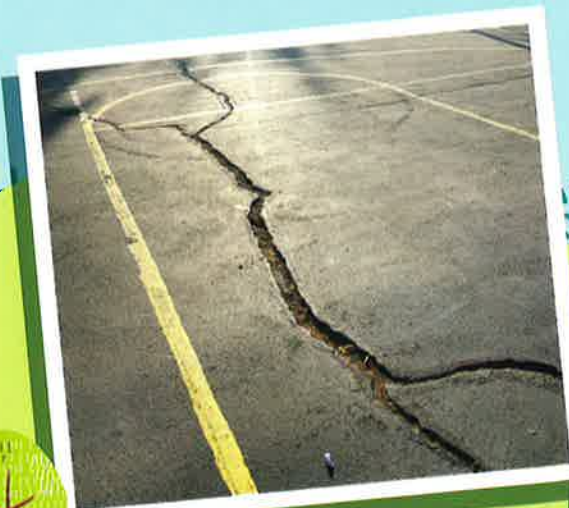
Hazardous cracks and uneven surfaces
